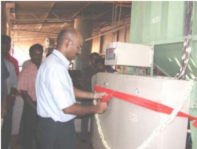
Mr. Senthil Kumar, CEO, S&V Industries, Akron, USA is inaugurating the newly installed dosing system.
