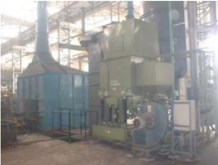
Newly commmissioned Sand Reclamation plant.
