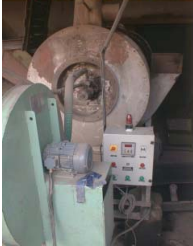
LPG Based sand drying system
