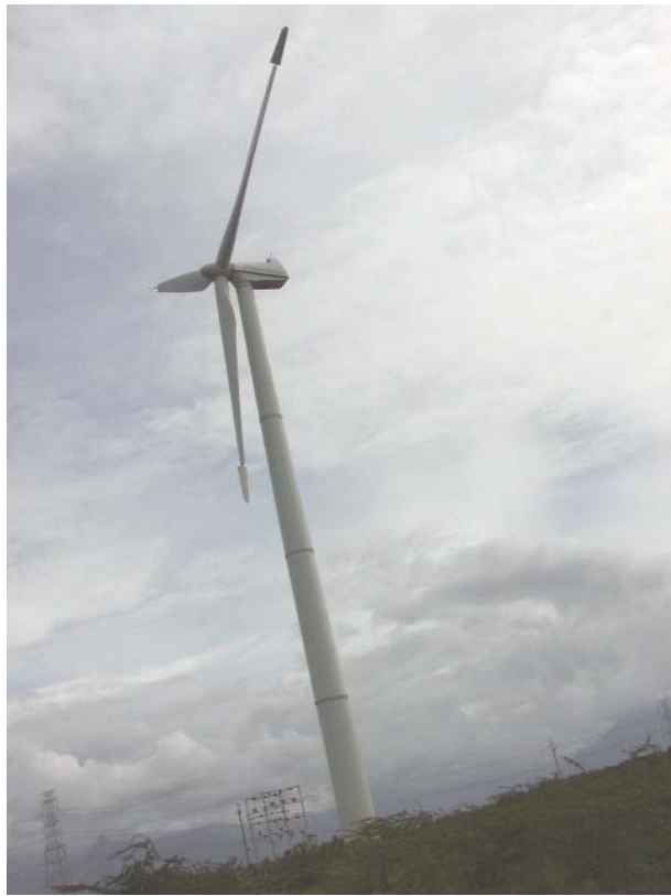
750 KW Wind Electric Generator
