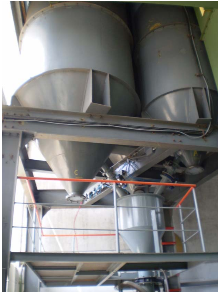
Sand Storage Hoppers
