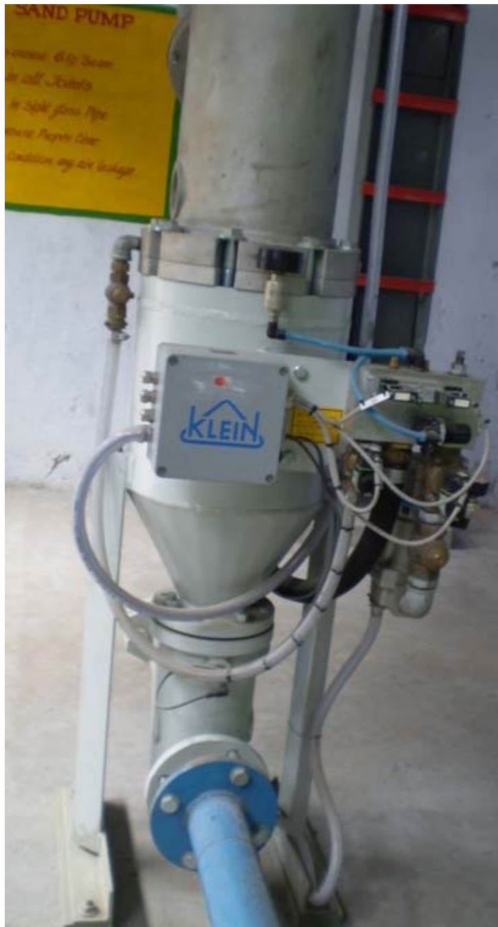
Sand Pumping System
